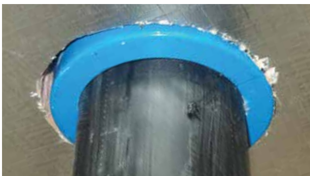
Figure 7 Penetration example - Kingspan Kooltherm™ K10 Soffit Board installed tight around the fire collar and HDPE service pipe.
